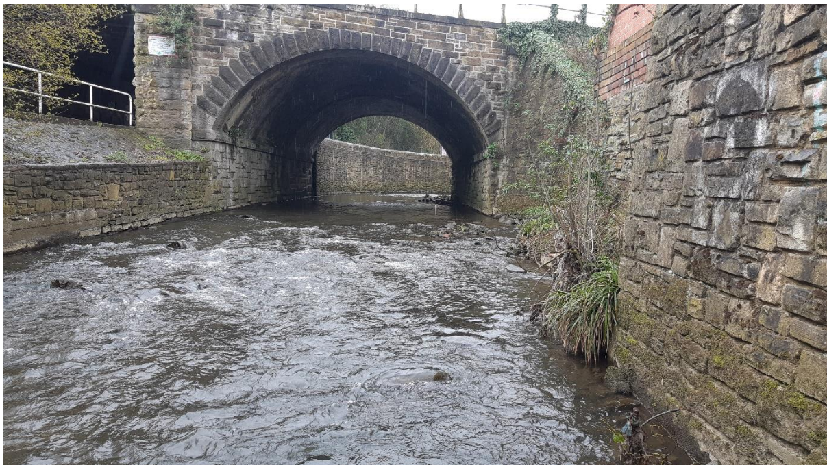
Figure 24: Boulder riffle below a bend pool and glide. Some vegetation colonisation of the rougher block stonework was evident here.
