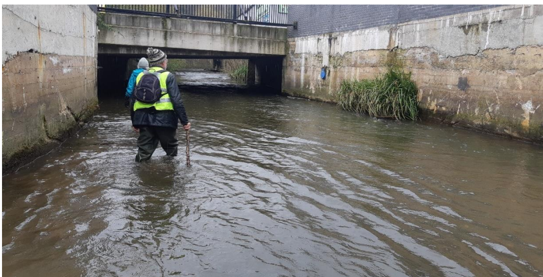
Figure 22: A clump of what appears to be pendulous sedge established in narrow cracks in the concrete (right of frame).
