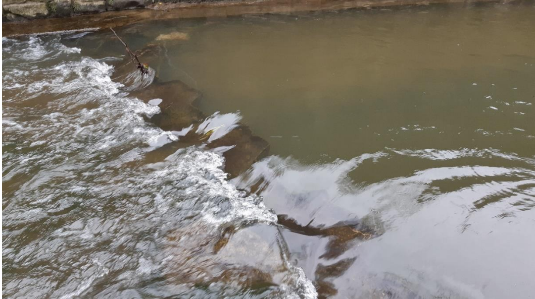
Figure 25: Sheet pile weir at 53.353558, -1.483511. Notching down to bed level of the central third (as a minimum) or complete removal should be investigated.
