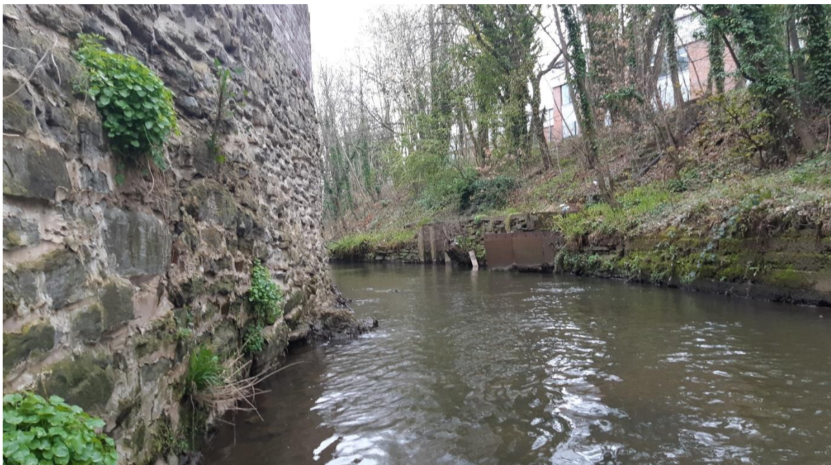
Figure 12: Walled channel with box-shaped wetted cross-section. The ecological value of patches of mature woodland is magnified by the extent of engineered modifications to the river.
