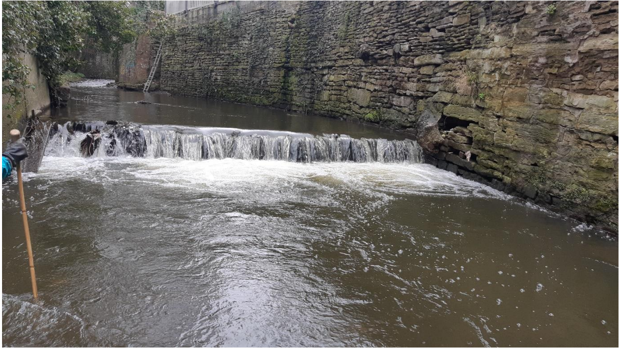
Figure 13: Sheet piling weir at 53.356944, -1.483056. Proposals to notch or remove the weir need to investigate whether walls within the impounded reach rely on hydrostatic pressure from the river for stability. Again, the existing erosive forces amplified by a barrier placed perpendicular to the walls should be incorporated into decision-making.
