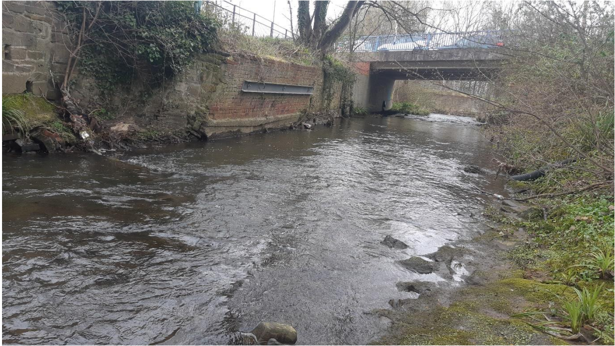
Figure 2: Facing downstream towards the downstream limit and the brick wall on the LB is clearly leaning over at a steep angle.
