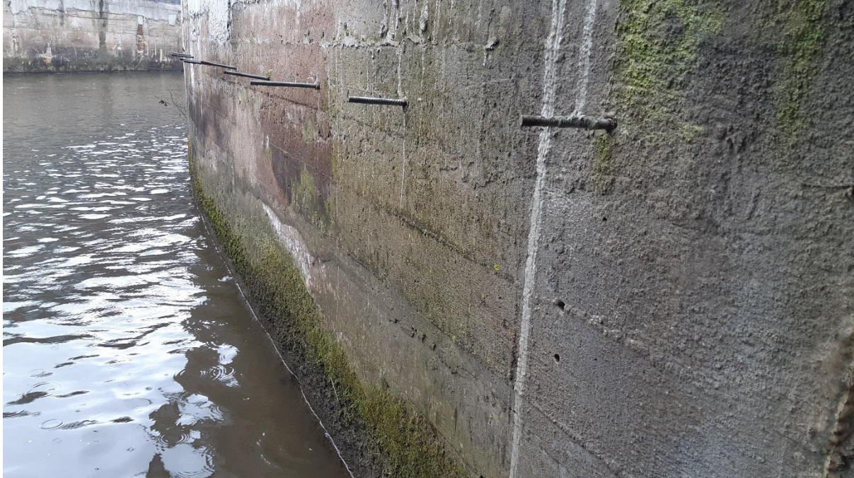
Figure 23: Protruding threaded bar ties were common throughout the concrete-walled section as far upstream as 53.354387, -1.483811.
