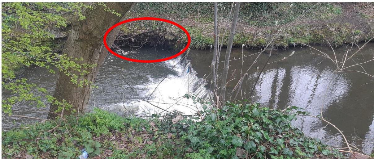
Figure 9: Sheet piling weir impounding a significant upstream reach and eroding the foot of the steep RB (ringed in red). This pattern of erosion is typical when barriers are installed perpendicular to the bank. While this could naturally bypass the weir, the bank supports a path and associated infrastructure. The weir is a barrier to up and downstream migration as well as a trap for substrate on its upstream side. Interventions could deliver ecological and local infrastructure benefits.
