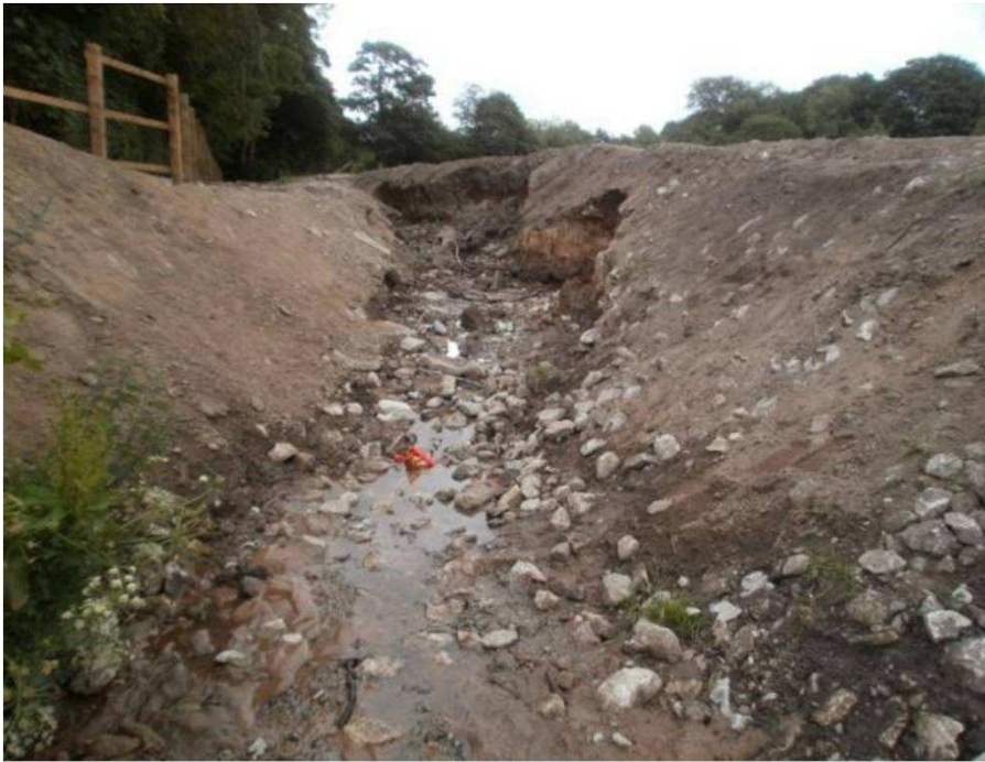
Photo 1: Before - Eroded channel before
