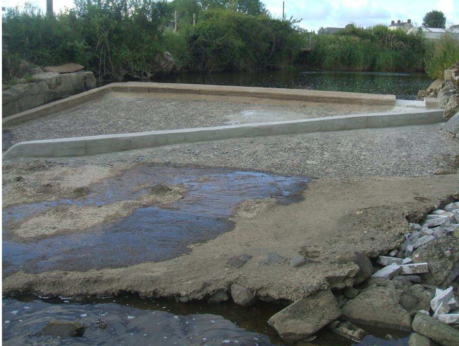
Figure 8: Diagonal baulk fitted to a sloping-faced (crump) weir. Structure is pictured in the dry with flow passing down an existing bypass channel to the left of frame. Could also be constructed using bolted wooden sleepers (cost - cement and metal pins)
