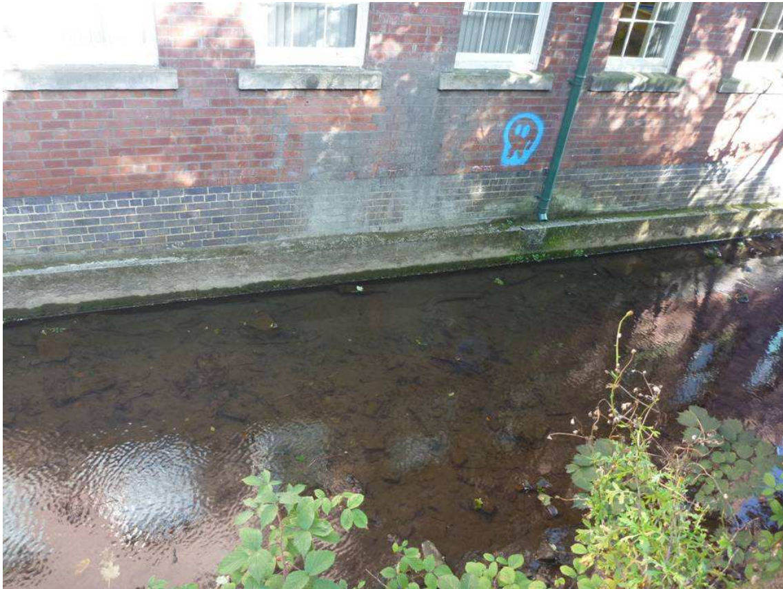
Figure 4: Overwide straightened section. There is a severe lack of overhead cover from predation here - along with a lack of deeper pool habitat. Both features would be required by adult fish. Deposition of fine sediments is also favoured from bank to bank. Such uniform deposition tends to reduce the variety of available microhabitats for both flora and fauna (although the presence of a variety of larger rocks is a valuable mitigating feature).
