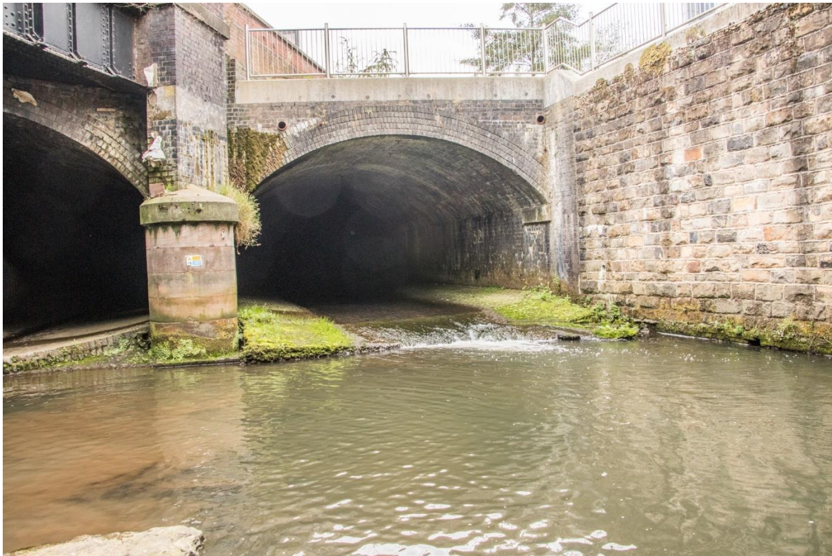
Figure 10: Double-arched ceiling, perched parallel culverts discharging into the short open-air section of the Sheaf at Ponds Forge. At low discharges, the only appreciable flow comes down the chamber on the right of this picture. However, the steep entrance and very shallow, laminar flow is in itself extremely difficult for fish to pass.
