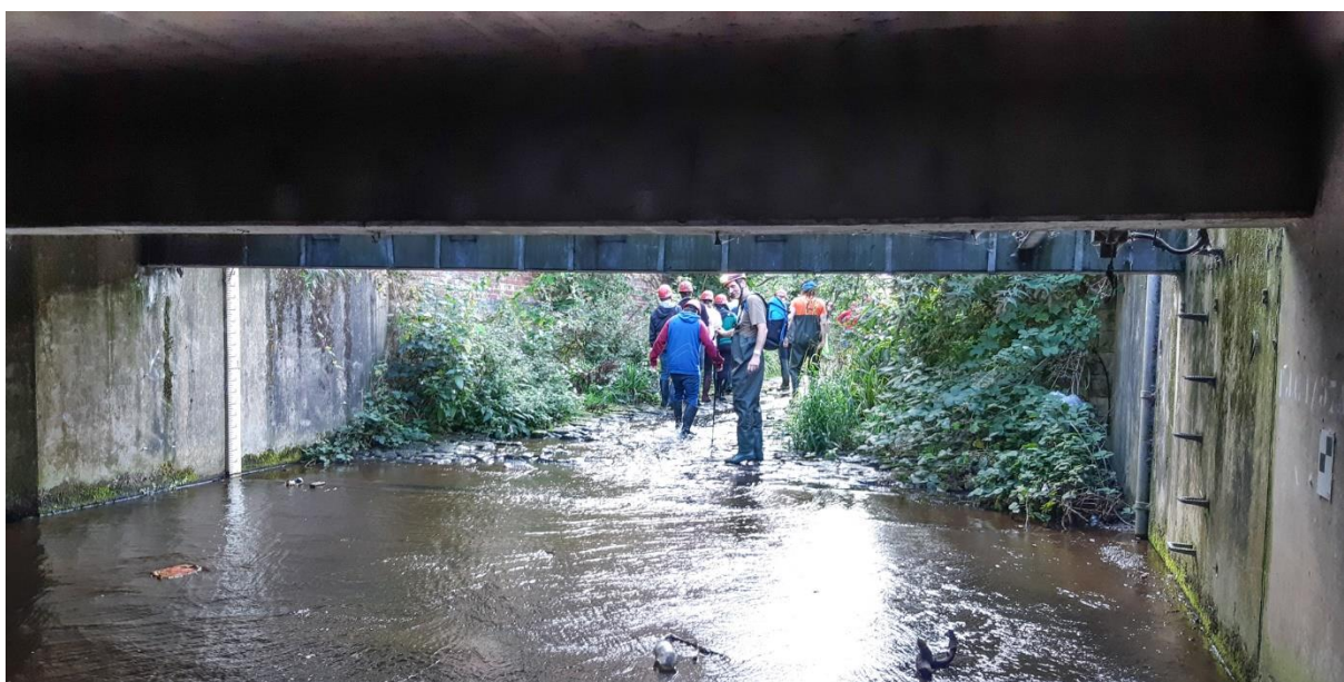
Figure 4: Culvert entrance at the junction between the reach adjacent to the Q-Park site and Sheffield Station.
