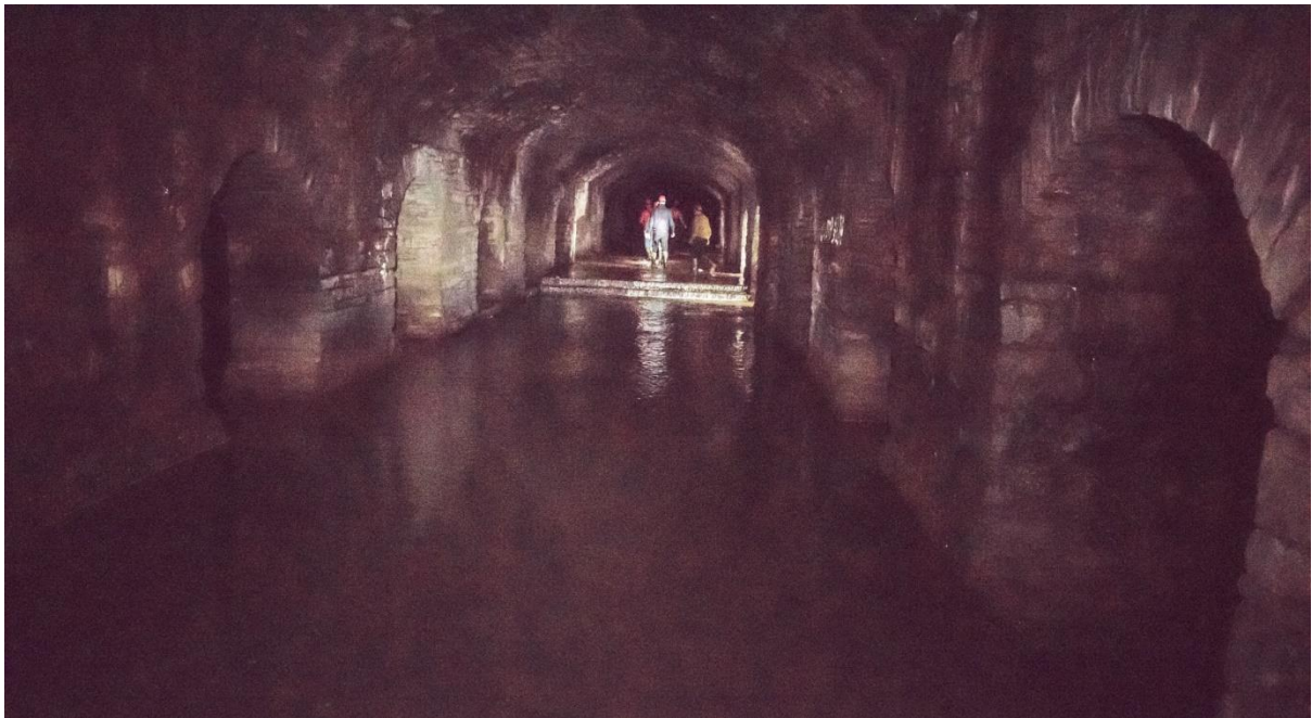
Figure 8: Archways to the left and right of frame can allow flow to pass down the culvert on either side.
